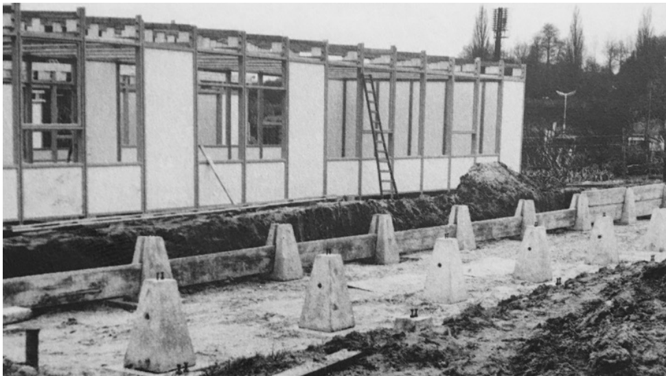
School pavilions' build-up, arch. Willy Van Der Meeren & Léon Palm (1957) concrete non-foundation + steel base + wooden upper structure + fiber panel finishing
